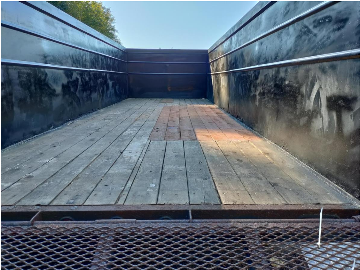
Figure 6. Boom trailer after rust treatment and floorboard replacement. Photo credit: Jeff Solomon
