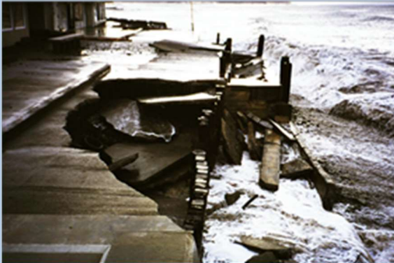
Coastal Flooding Damage at Sandy Point in 2000
